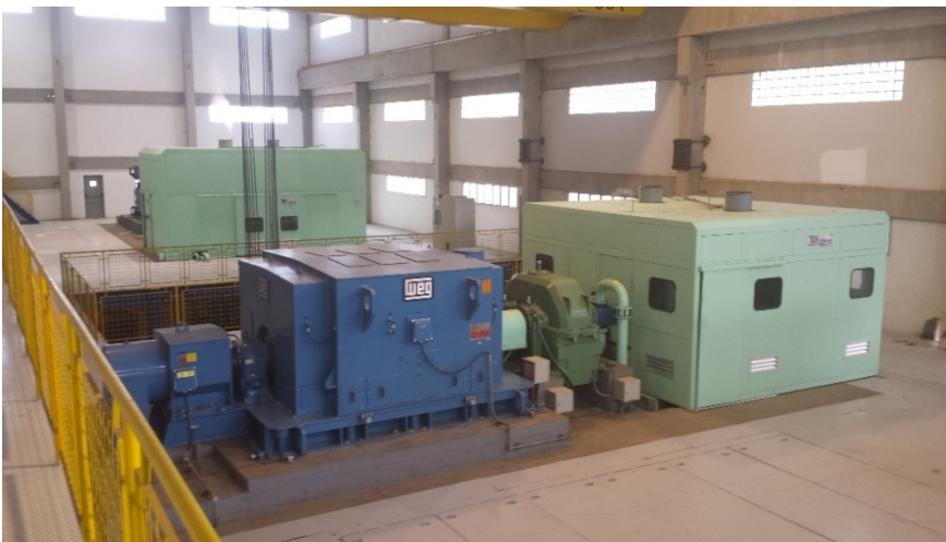
Power Generator 1 and 2
