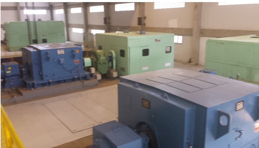
Power Generator 1, 2 and 3
